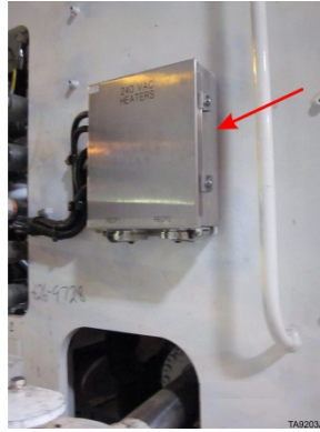
Component heater connection box is located within articulation area-left side of machine.
